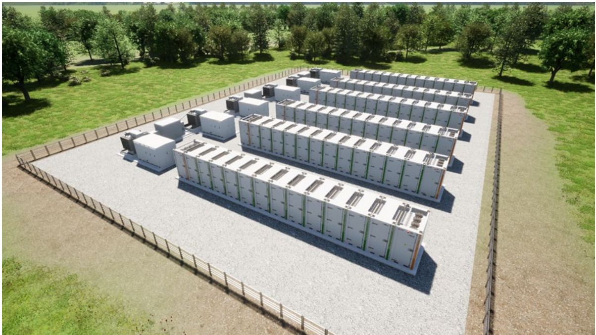
Image 3.6 Typical BESS Units
